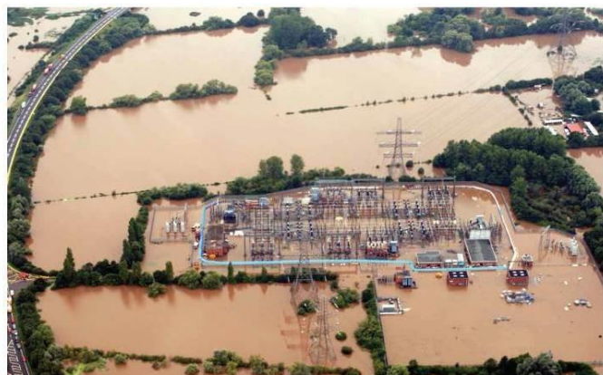
Walham electricity transmission switching centre
