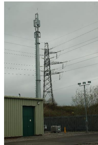
400 MHz utility LTE system
