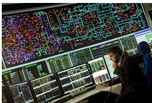
National Grid control room illustrating the dependence of electricity grids on telecommunications to enable them to operate their networks.
