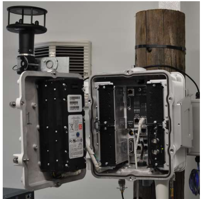
Device Power: Mission critical devices may require back-up power in case of loss of mains supply. Batteries in the cover of this pole-mounted telemetry device guarantee continued operation for a minimum of 72 hours after the loss of mains power.
