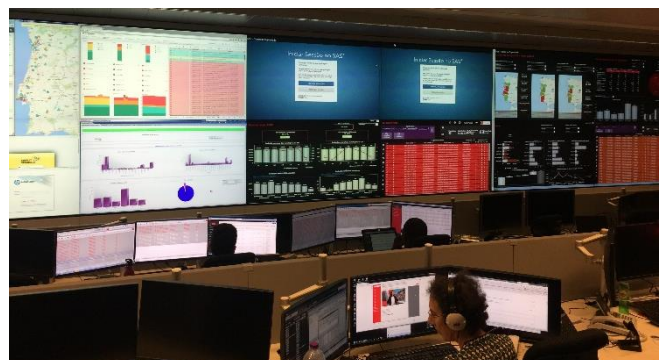
Typical utility distribution control room
