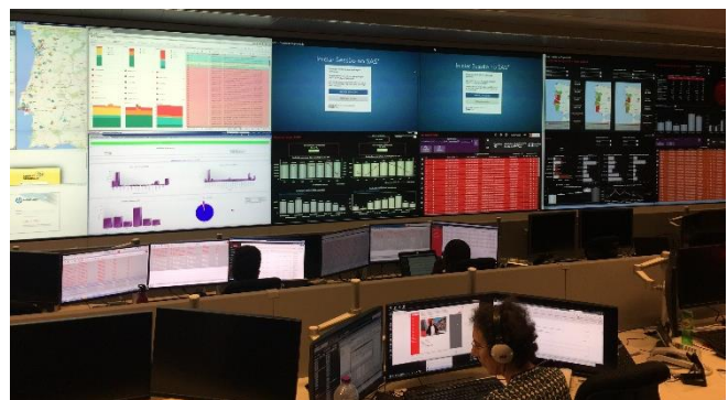
Typical utility distribution control room
