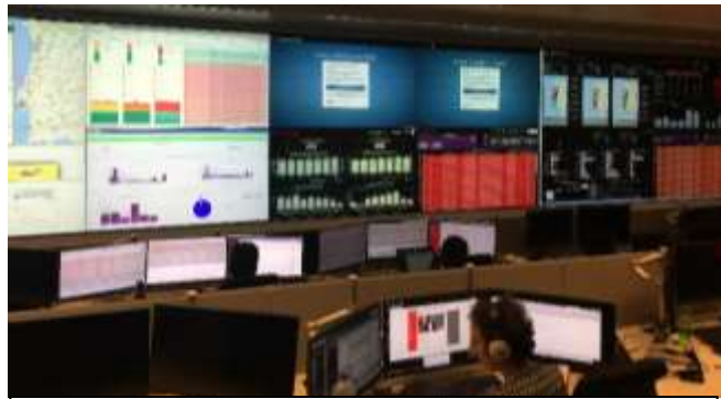
Typical utility distribution control room
