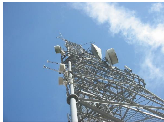
Utility radio tower
