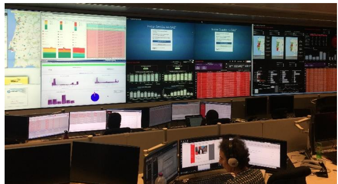
Typical utility distribution control room
