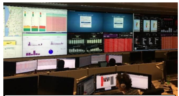
Typical utility distribution control room
