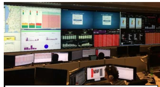
Typical utility distribution control room
