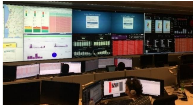
Typical utility distribution control room
