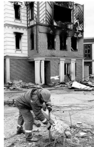
12% of all power lines in Ukraine have been damaged since 2022
