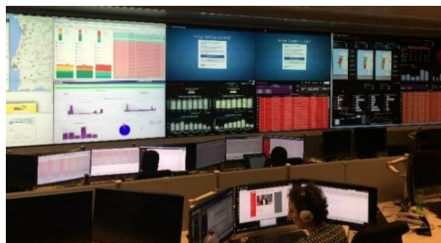
Typical utility distribution control room
